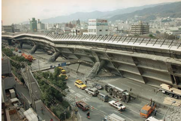
Fig. 1. Failure of a flyover on the “Hanshin” expressway after the 1995 Kobe earthquake source: https://www.japantimes.co.jp/opinion/2020/01/16/editorials/learned-enough-1995-kobe-quake/
