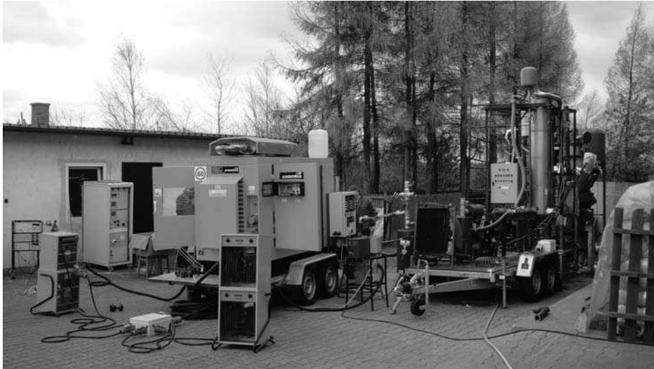
Fig. 1. The generating set connected to the gasification installation during the indication of the double-fuel engine [3]
